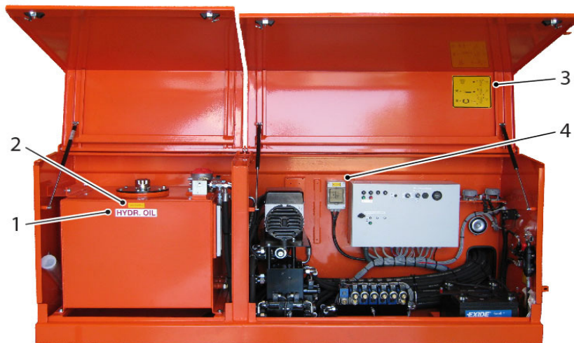
Hydraulic oil and valve/electrical compartment
